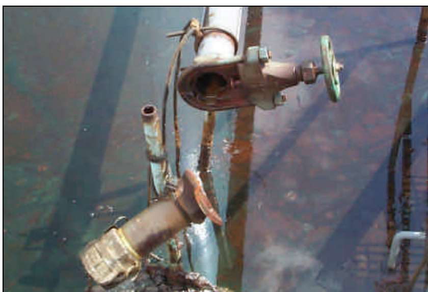
Broken valve can result in contamination
