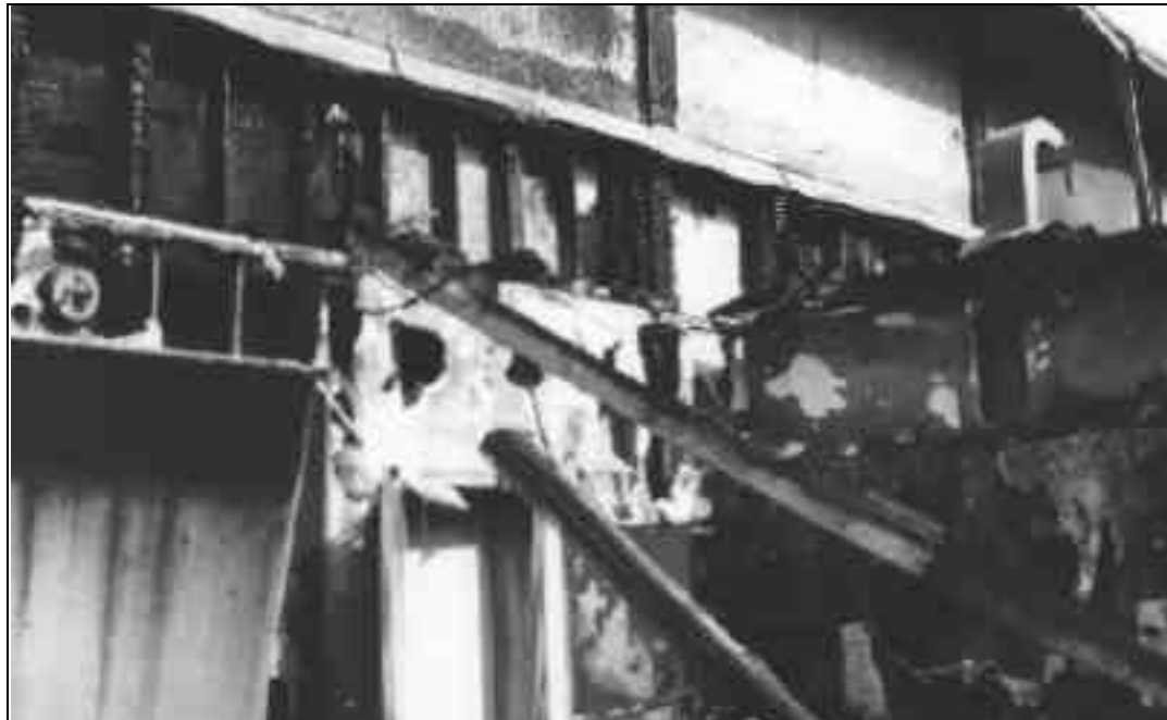
Damage from fire at Seaview Elementary School, Lantzville, October 6, 1994
